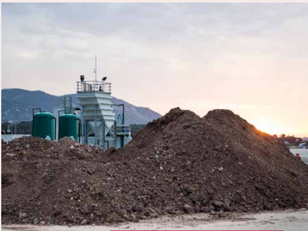
The contaminated sediments are sorted into sand and fine clay. The sand fraction is decontaminated and re-used.
