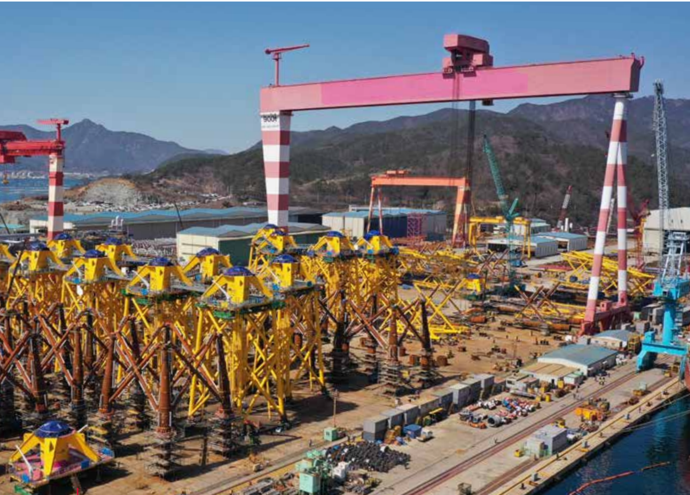
Jan De Nul Group was responsible for the construction of the Taiwan Power Windfarm Phase 1 Project – Demonstration in Changhua. From the design over the construction of the foundations and their transport up to the installation of the foundations, the onshore and inter array plus export cables, the onshore substation and the wind turbines.
