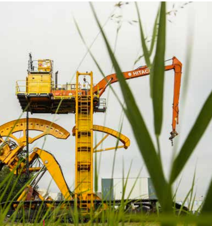
This in-house designed machine digs in cables into the ground in an intertidal area. The earth pressure of the machine is smaller than that of a person so that it can even be deployed in nature reserves.
