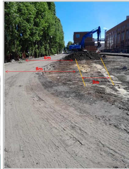
Figure 11: Location of 8 kV Cable
