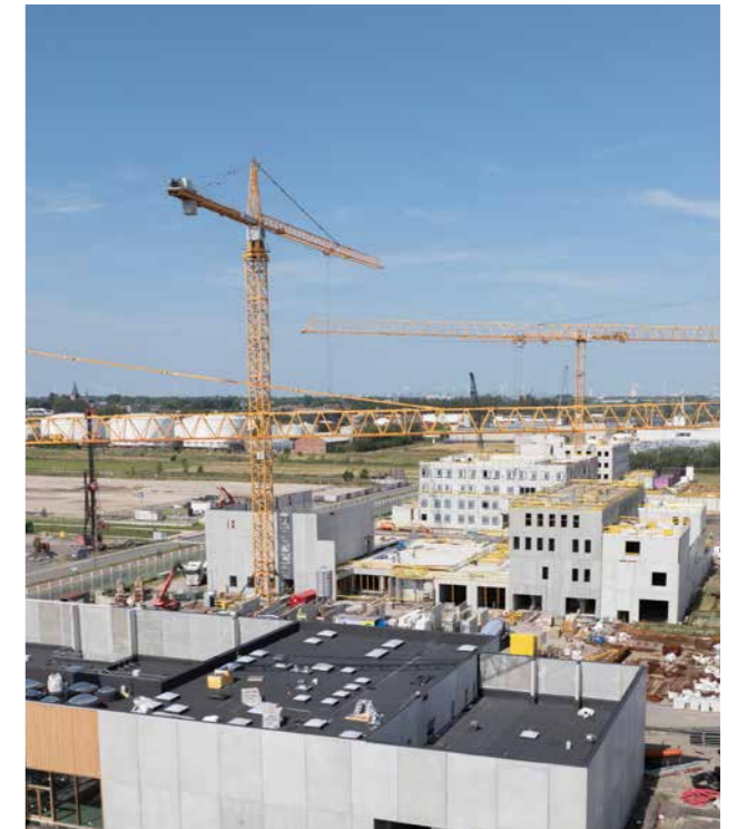
Together with our partners, we are responsible for the design, construction, financing and maintenance of Antwerp's new prison, set to house 440 inmates from mid-2026.
