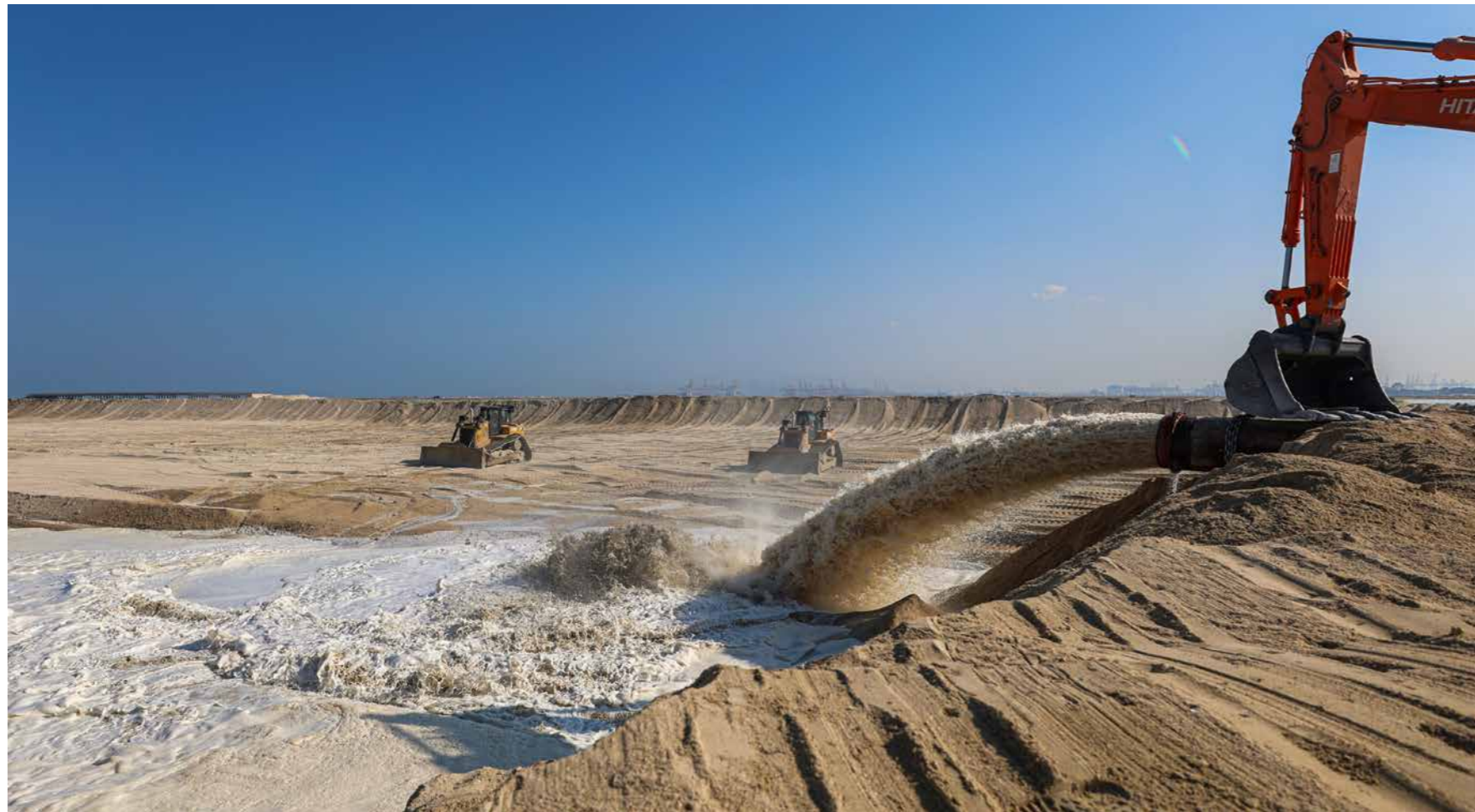
In Dubai, we constructed Palm Island II, a world-class tourist venue to stress the region's reputation in unique holiday experiences. This artificial peninsula has the shape of a palm tree, with 16 palm leaves each 80 metres wide.
