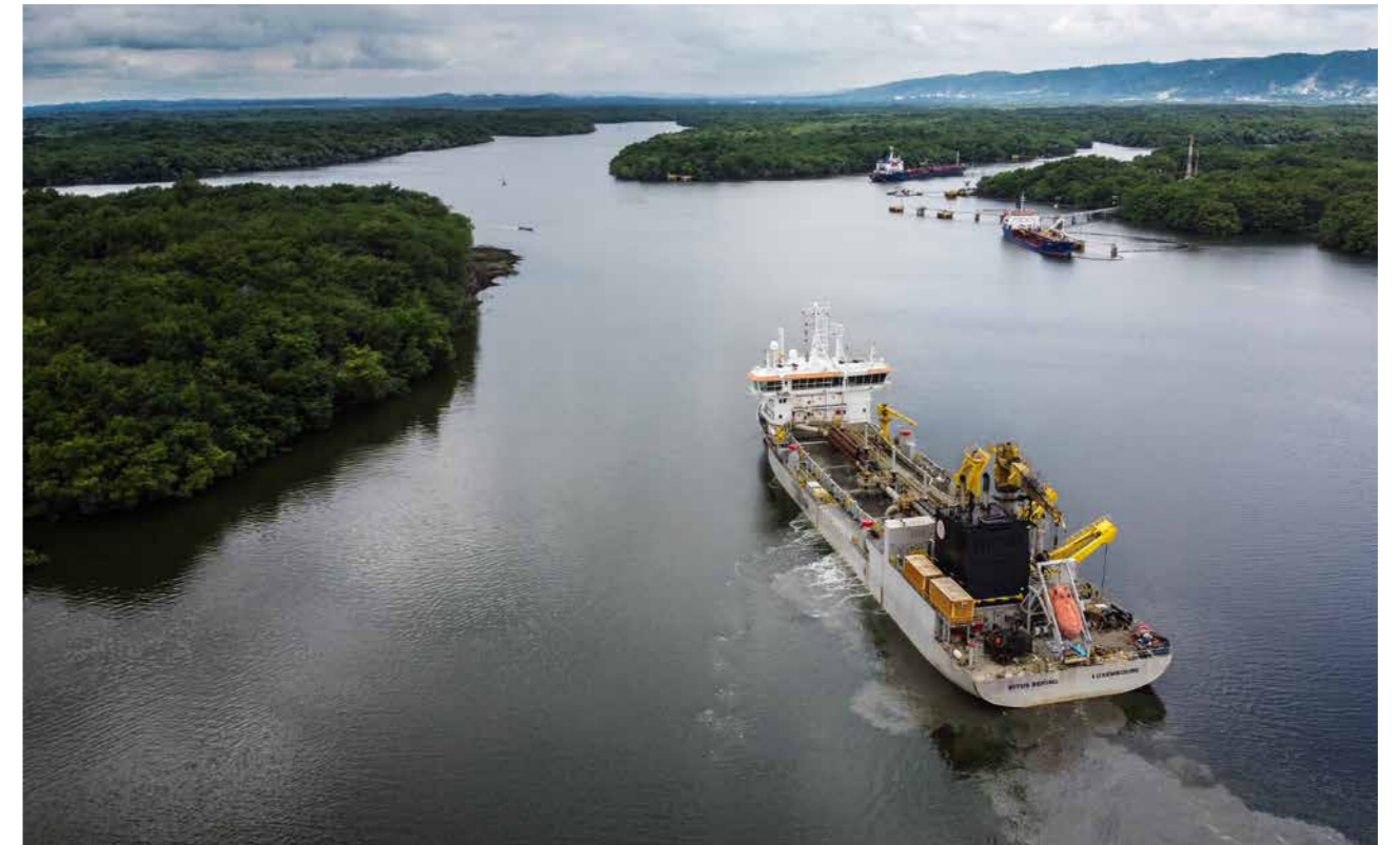
To keep the port of Guayaquil, Ecuador, accessible to Neo Panamax and other large vessels, we deepened its access channel to 12.5 metres.
