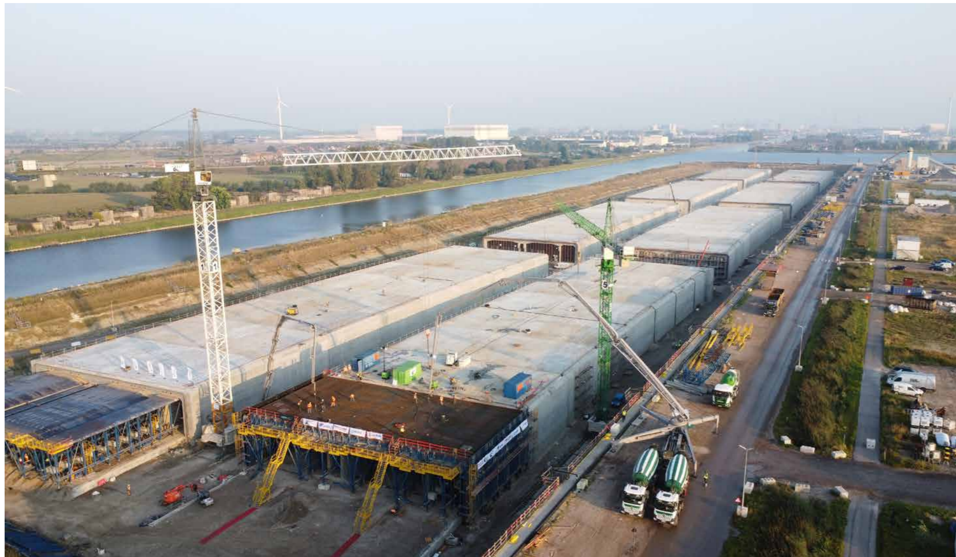
To reduce traffic density in Antwerp, we are constructing a 1.8-km tunnel between the left and right bank of the Scheldt river, with three lanes in each direction.
