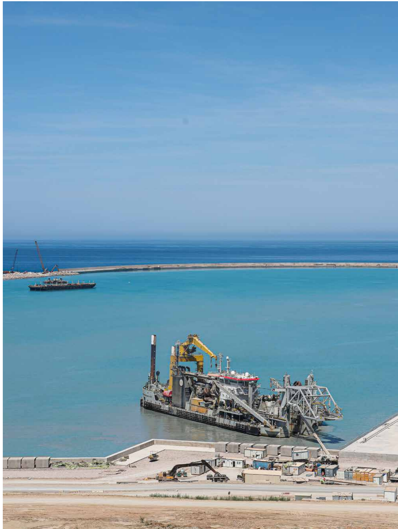
In the Tangier-Tetouan region, Morocco, we constructed a brand-new deep-water port with an integrated industrial platform and free-trade zone.
