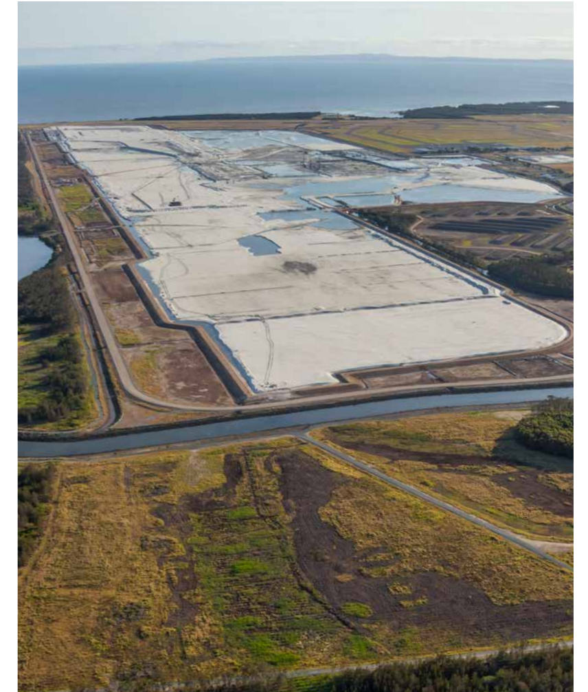
For the Brisbane Airport, Australia, we reclaimed a 300-hectare platform for the construction of a new runway.
